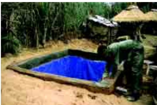
Plate 2.5 Rectangular tank with polythene lining.
